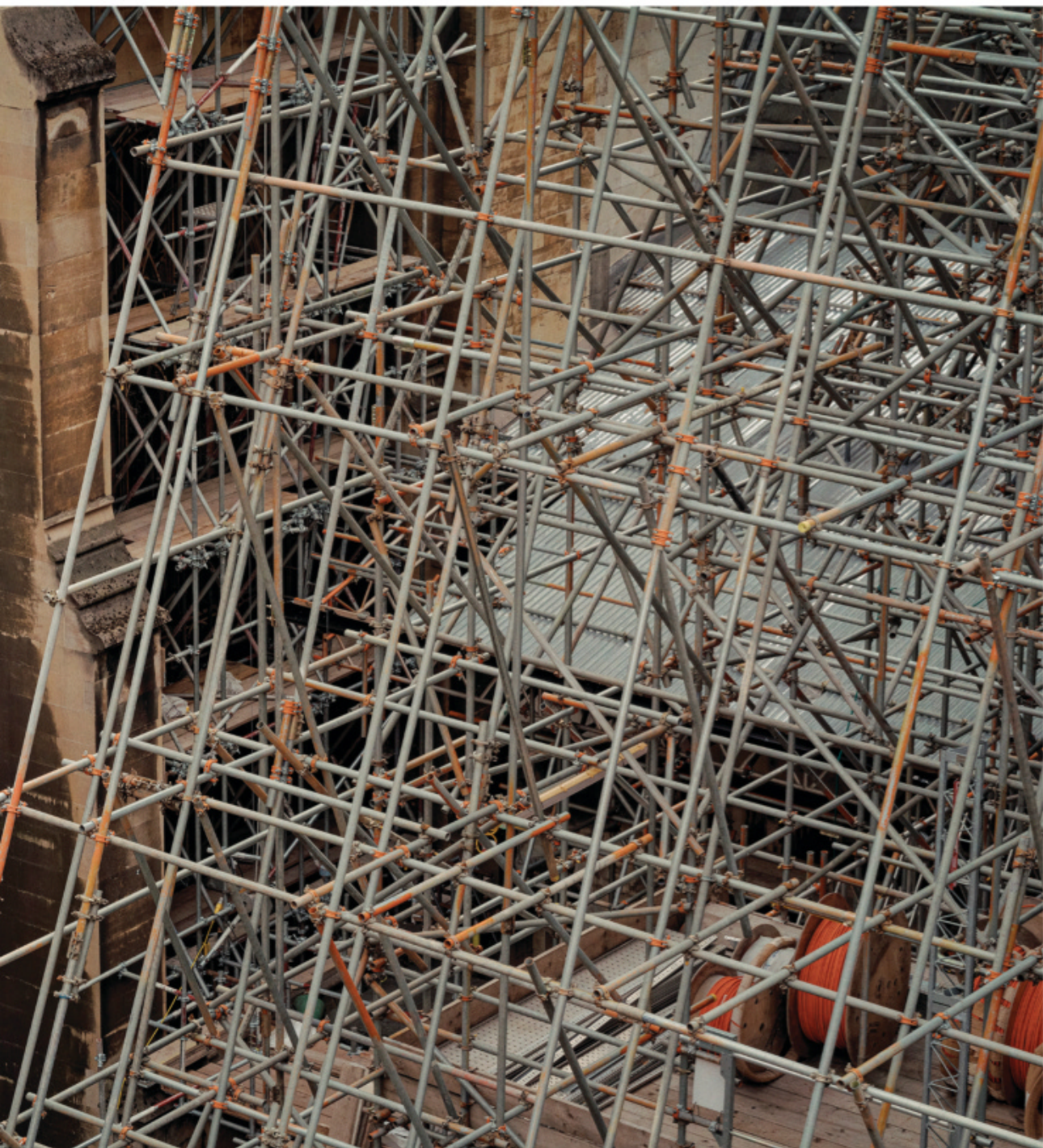
^ Scaffolding covers much of the palace's blackened walls, partly to protect people from falling stone
