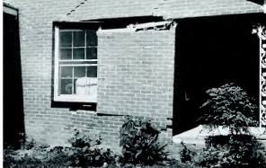
Figure 11.37 Cracked outside wall in a home built on clay-rich soils. This house was severely damaged because the surrounding soil contains expandable clays, which can either expand like a sponge when wet or lose cohesion and collapse when they dry.
