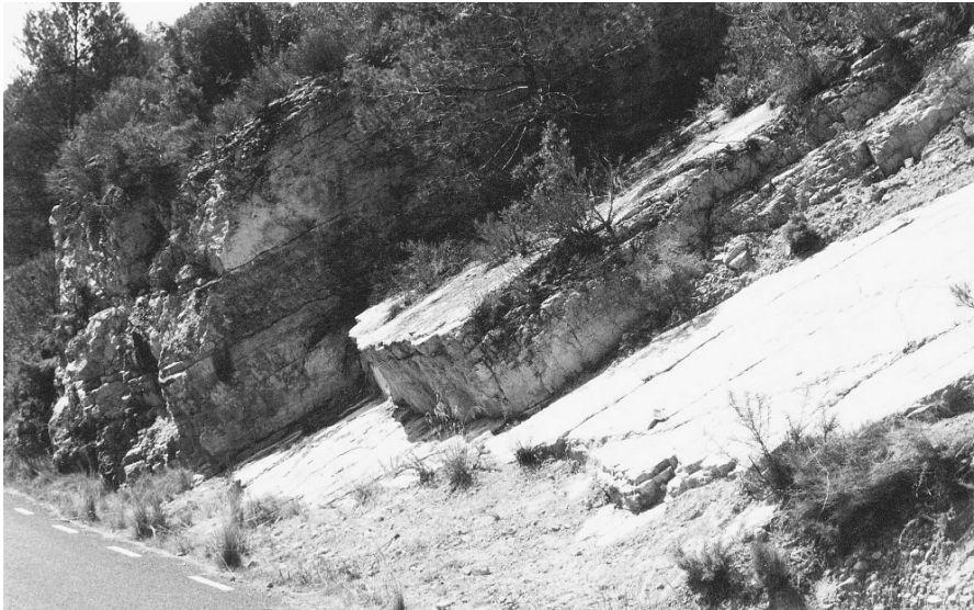
Fig. 3.1. Bedding planes as mechanical discontinuity planes causing failure of a slope in limestone
