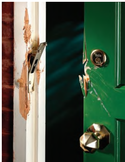
Figure 16-2. Indentation: Screwdrivers often make a nick or impression in a surface they are used on.
