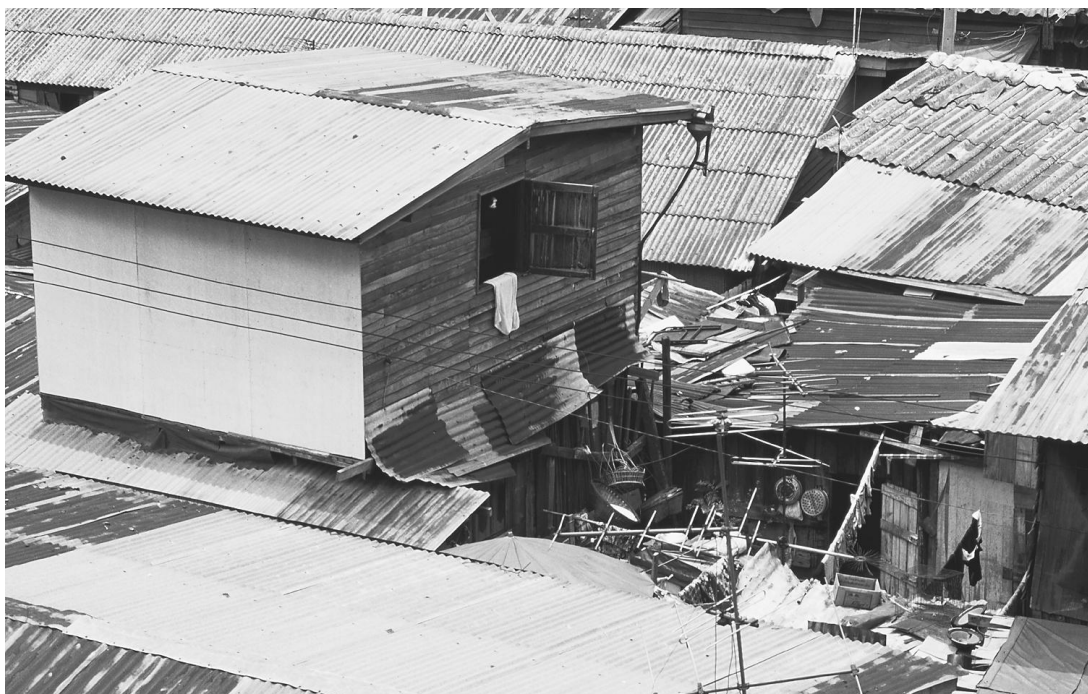
MOST “TIN” ROOFS NOW CONSIST OF AN IRON OR STEEL ROOF COVERED WITH ZINC, NOT TIN. (John Hulme; Eye Ubiquitous/Corbis. Reproduced by permission.)
