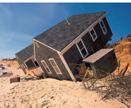
FIGURE 5.19 Winter storms have eroded the beach and undermined the foundations of homes on this barrier island. Breaking through protective dunes to build such houses damages sensitive plant communities and exposes the whole island to storms and erosion. Coastal zone management attempts to limit development on fragile sites.
