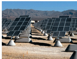
(c) Base-load solar power facility
