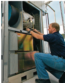
FIGURE 20.8 A technician adjusts a gas microturbine that produces on-site heat and electricity for businesses, industry, or multiple housing units.
