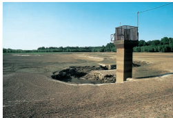
FIGURE 17.21 This dam is now useless because its reservoir has filled with silt and sediment.
