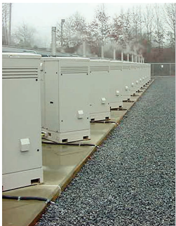
FIGURE 20.17 The Long Island Power Authority has installed 75 stationary fuel cells to provide reliable backup power.
