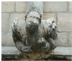
FIGURE 16.23 Atmospheric acids, especially sulfuric and nitric acids, have almost completely eaten away the face of this medieval statue. Each year the total loss from air pollution damage to buildings and materials amounts to billions of dollars.
