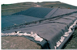
FIGURE 21.7 A plastic liner being installed in a sanitary landfill. This liner and a bentonite clay layer below it prevent leakage of groundwater. Trash is also compacted and covered with earth fill every day.
