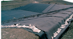
FIGURE 21.7 A plastic liner being installed in a sanitary landfill. This liner and a bentonite clay layer below it prevent leakage to groundwater. Trash is also compacted and covered with earth fill every day.
