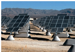
(c) Base-load solar power facility
