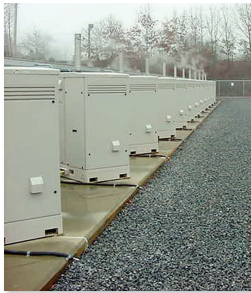
FIGURE 20.17 The Long Island Power Authority has installed 75 stationary fuel cells to provide reliable backup power.
