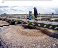
FIGURE 18.23 In conventional sewage treatment, aerobic bacteria digest organic materials in trickling filter beds in high-pressure aeration tanks. This is described as secondary treatment.
