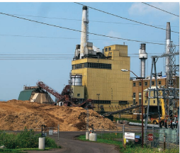
FIGURE 20.18 This Michigan power plant uses wood chips to fuel its boilers. Where wood supplies are nearby, this is a good choice both economically and environmentally.
