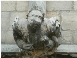
FIGURE 16.23 Atmospheric acids, especially sulfuric and nitric acids, have almost completely eaten away the face of this medieval statue. Each year the total loss from air pollution damage to buildings and materials amounts to billions of dollars.
