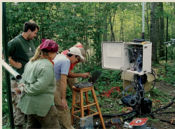
FIGURE 2.2 A student researcher adjusts the electrical panel that controls heat lamps and heating cables.
