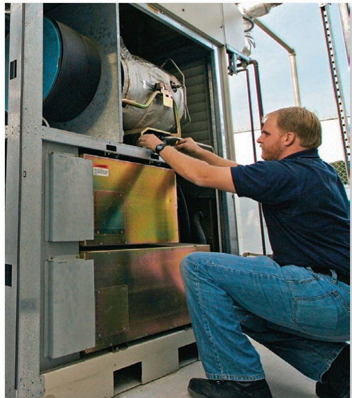
FIGURE 20.8 A technician adjusts a gas microturbine that produces on-site heat and electricity for businesses, industry, or multiple housing units.
