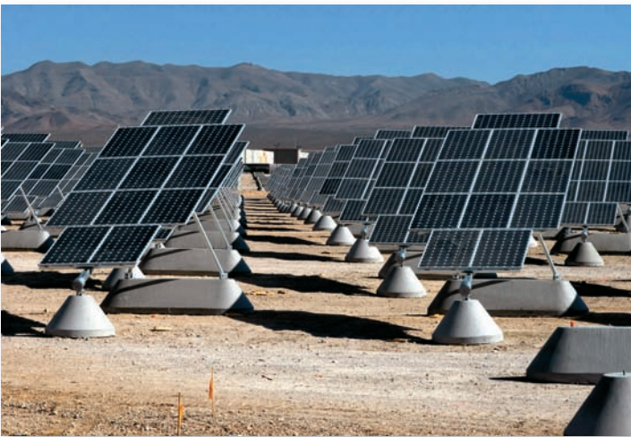
(c) Base-load solar power facility
