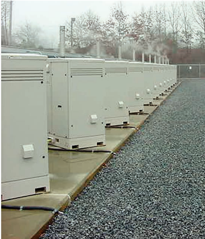
FIGURE 20.17 The Long Island Power Authority has installed 75 stationary fuel cells to provide reliable backup power.
