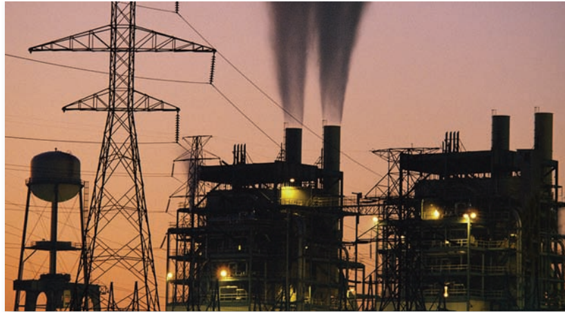
FIGURE 16.3 Primary pollutants are released directly from a source into the air. Coal-burning power plants like this one produce about two-thirds of the sulfur oxides, one-third of the nitrogen oxides, and one-half of the mercury emitted in the United States each year.
