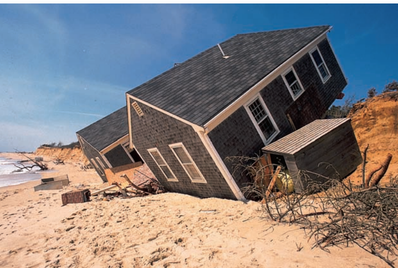
FIGURE 5.19 Winter storms have eroded the beach and undermined the foundations of homes on this barrier island. Breaking through protective dunes to build such houses damages sensitive plant communities and exposes the whole island to storms and erosion. Coastal zone management attempts to limit development on fragile sites.
