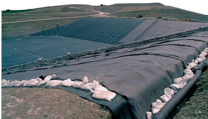
FIGURE 21.7 A plastic liner being installed in a sanitary landfill. This liner and a bentonite clay layer below it prevent leakage to groundwater. Trash is also compacted and covered with earth fill every day.
